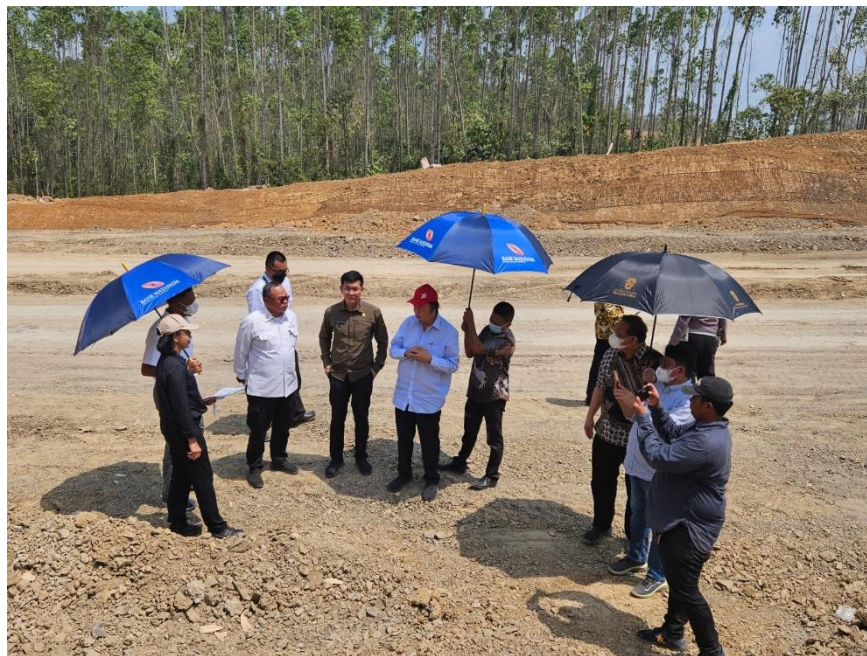
Dato Sri Tahir (center) together with representatives of the NCA inspected the construction site for the Mayapada Hospital in WP 1B Nusantara, on Tuesday (03/10/2023).
